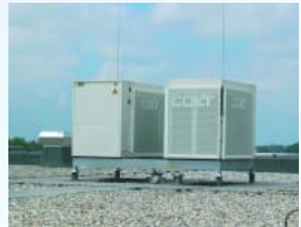
The external central heat pump installed at Nic. Oud Direct Mail, Holland
